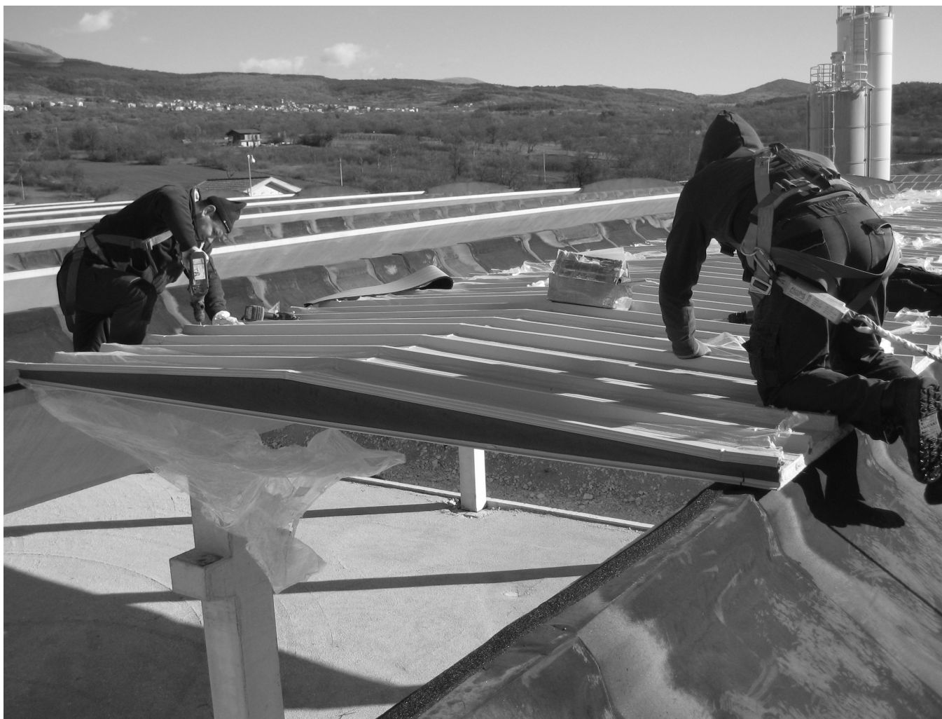
Picture n° 11: laying of the TECHTUM panel on reinforced concrete wing beams
