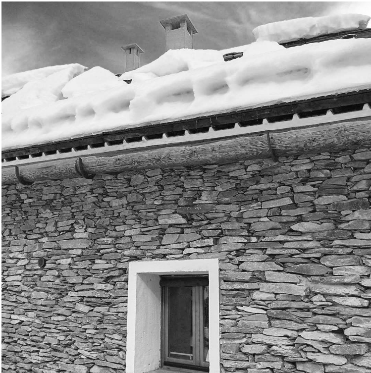
Picture n° 7: roofing of a refuge located in an Alpine area (2000 m asl) and made with sandwich panels on which wooden battens and shingles were laid.
